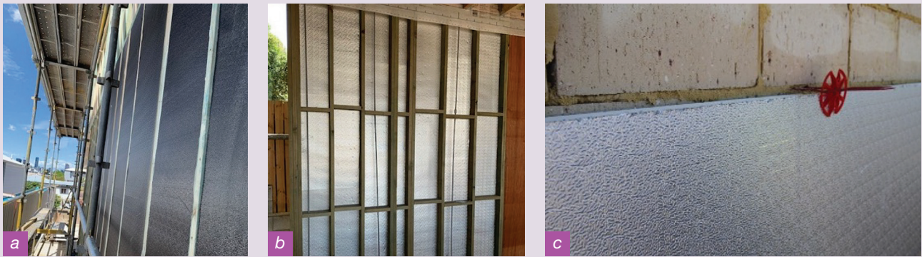
Figure 1: a) and b) Foil faced PIR insulation board installed external to the frame (continuous insulation) on a low-energy house in Brisbane prior to installing cladding (photos courtesy of Pirmax Pty Ltd), c) Foil faced PIR insulation board being installed in the cavity of a double brick construction (photo courtesy of Reflex Insulation Pty Ltd).
