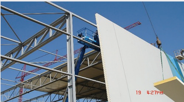
Figure 3: Large single storey warehouse being constructed from metal faced PIR composite panels (photo courtesy of Polyurethane Consulting Services Pty Ltd).
