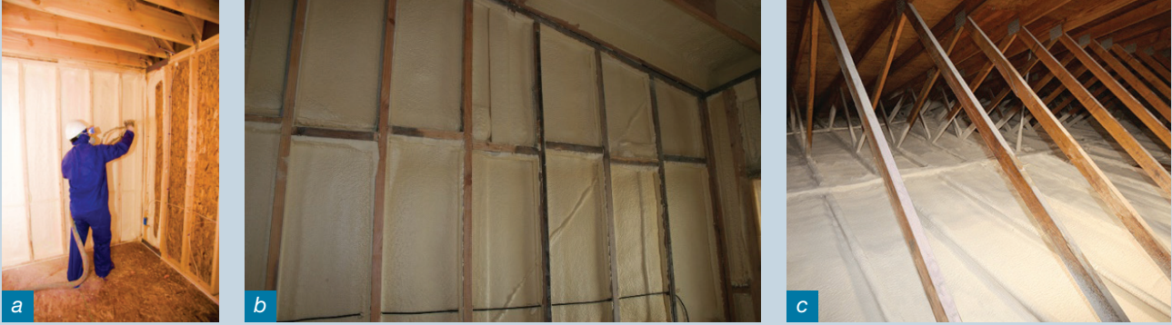
Figure 2: SPF applied in a timber frame house a) ocSPF in the USA, b) ccSPF sprayed between the wall studs in Melbourne Australia, c) ccSPF sprayed between the ceiling joists in the USA (photos courtesy of Huntsman Polyurethanes).
