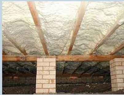
Figure 8: Application of ccSPF under a timber floor in Canberra (photo courtesy of Pacific Urethanes Pty Ltd).
