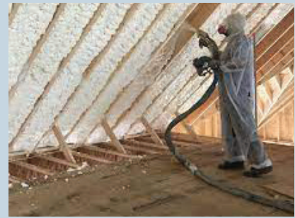
Figure 9: Application of ocSPF between the roof rafters prior to trimming the foam back to stud level (photo courtesy of Huntsman Polyurethanes).
