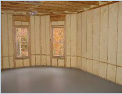
Figure 7: ocSPF applied between the wall studs to provide insulation and an air-barrier (photo courtesy of Huntsman Polyurethanes).
