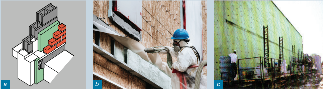
Figure 3: ccSPF applied to a concrete block wall with a brick veneer cladding (photos courtesy of Huntsman Polyurethanes).
